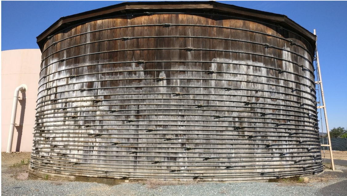
Figure 6. Condition of B Tank #1
