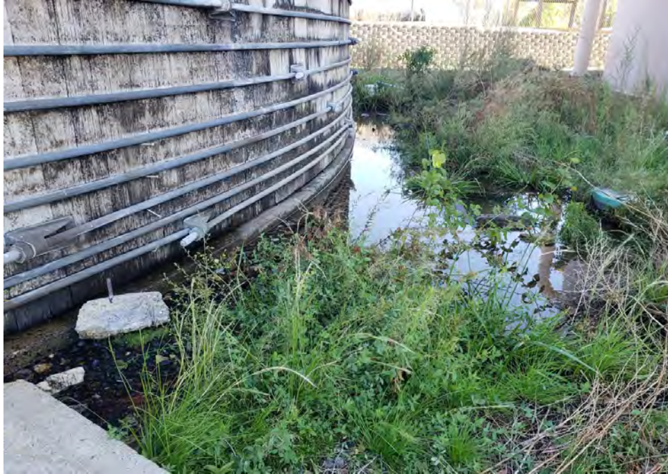
Overview showing series of metal bands and fasteners of redwood tank as well as obvious signs of leaking on tank's southeast side, facing east, taken 11/10/22, Photo #134610, from Photolog BS-01.
