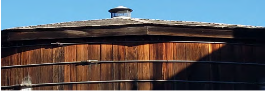
Close up #2 of redwood tank roof, showing small superstructure for ventilation and shingles, taken 11/10/22, Photo #135453, from Photolog BS-01.
