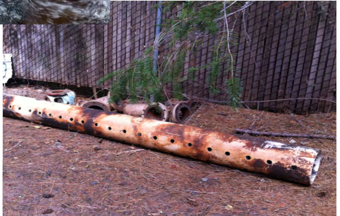
Middle Fork Mokelumne River Pump Station Intake
