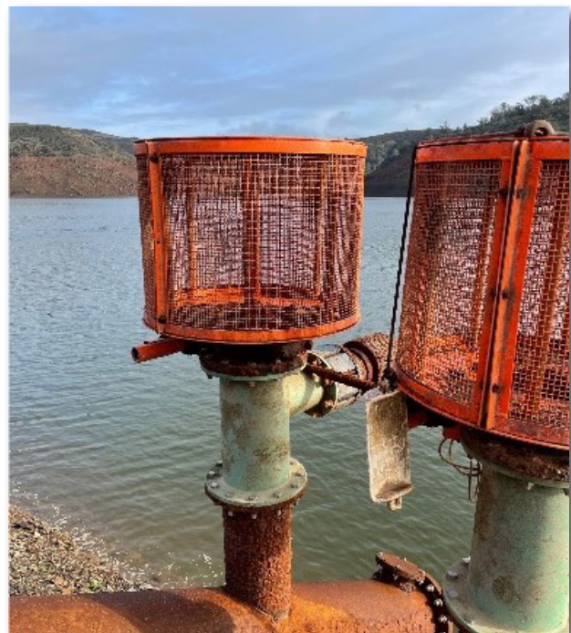
↑ FIGURE 3 - LAKE MCCLURE WATER INTAKES
